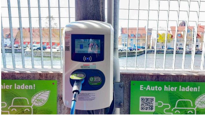
E-Auto Ladestation Parkhaus am Ozeaneum - © TZ HST
