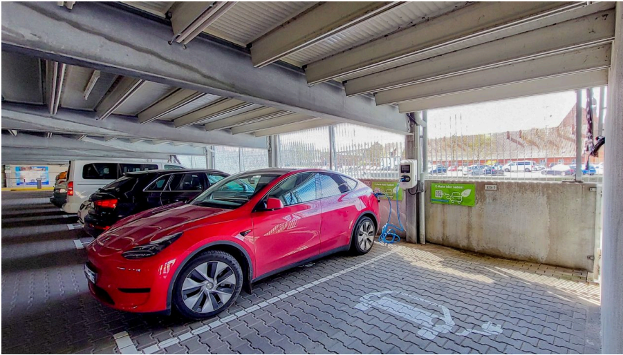
E-Auto Ladestation Parkhaus am Ozeaneum - © TZ HST
